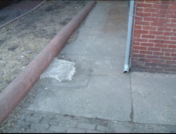
Covered up drain. Water now just pools.
