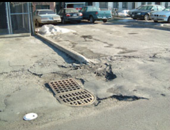
Parking lot with extra drain, showing massive water damage to asphalt.
